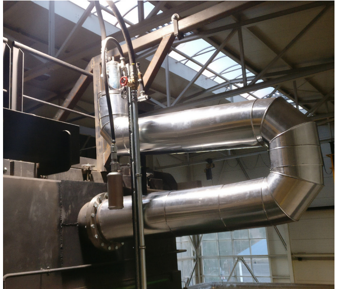
Smoke Tube Boiler - Äppelbo, Sweden
