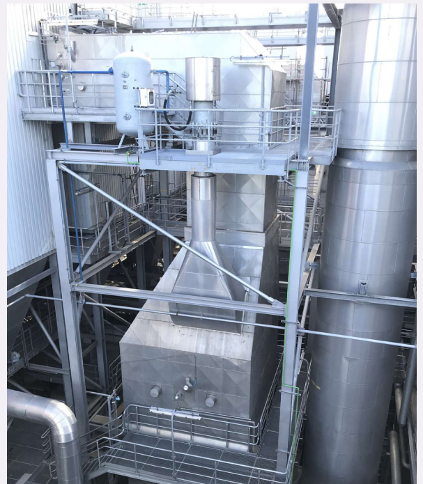
Infrasound Cleaner installed on a Waste-to-Energy Boiler
